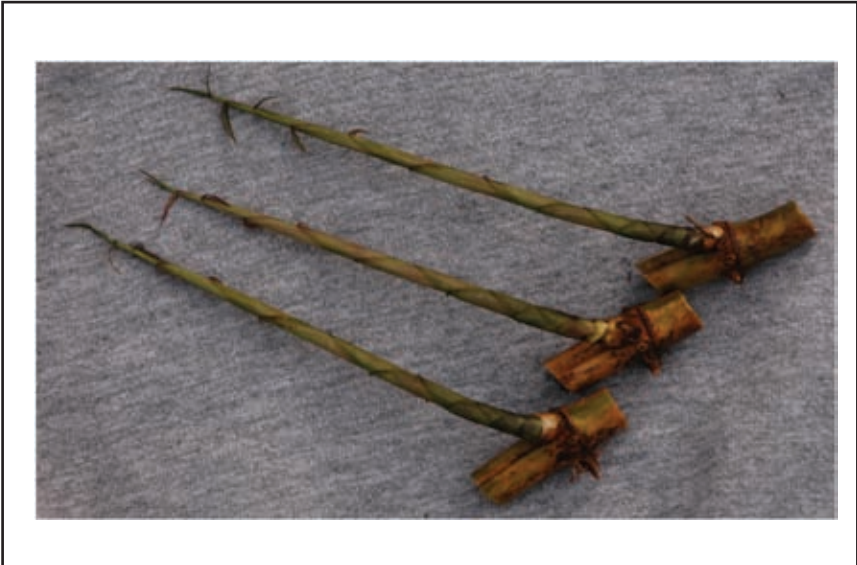
Figure 2. New bamboo culms and many grass stolons are sharp enough to penetrate the roof membrane.
