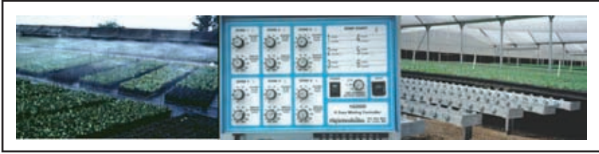
Figure 6. Static mist control systems rely on clocks and timers. They are unable to automatically respond to daily fluctuations in light irradiance, cloud cover, relative humidity, temperature, or stage of root development.
